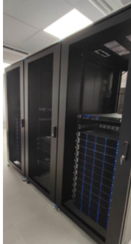
Figure 3: Cabinets with the RAEGE correlator equipment
