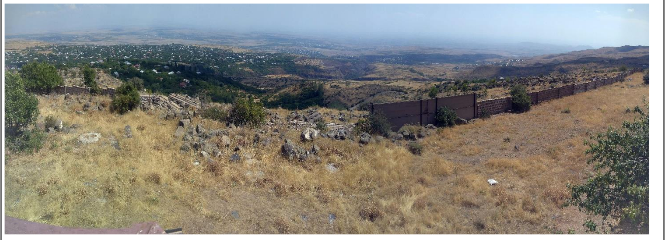
Picture 1 - One of the destroyed sections of the SCA fence
