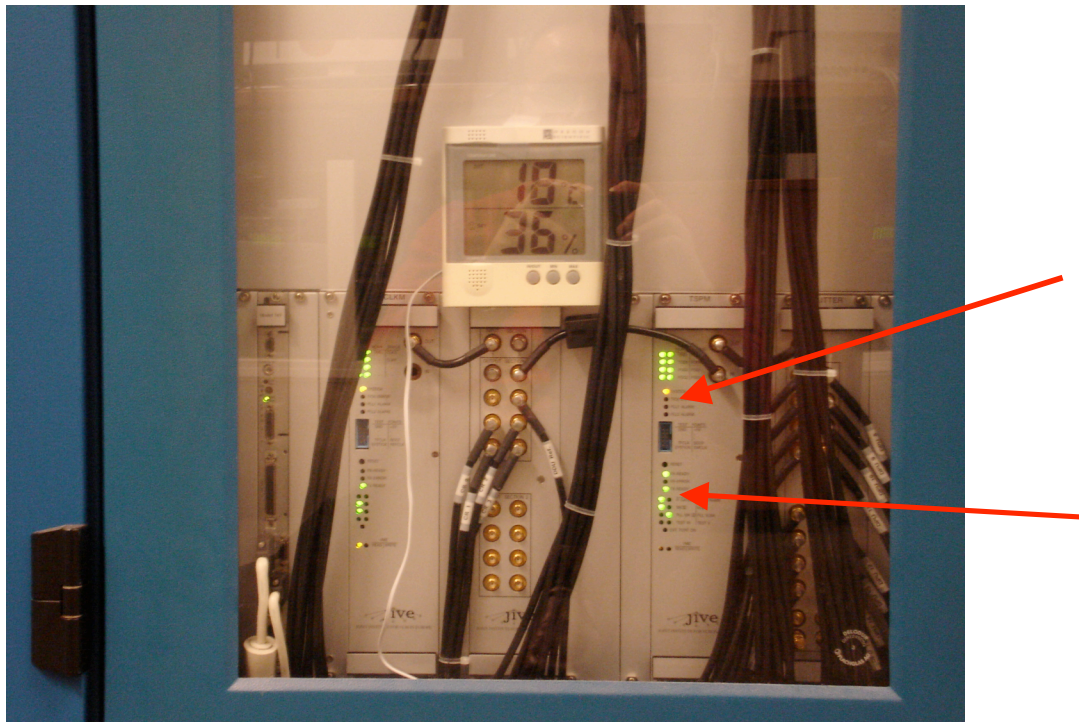
Picture 1: TSPU as it should look. Watch out for red leds at the positions of the arrows.
