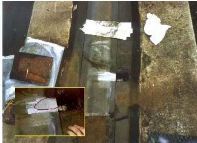
The cracked section of the Effelsberg azimuth track with a close up of the crack (insert, circled in red). Courtesy Richard Wielebinski. (click on image for larger version)
