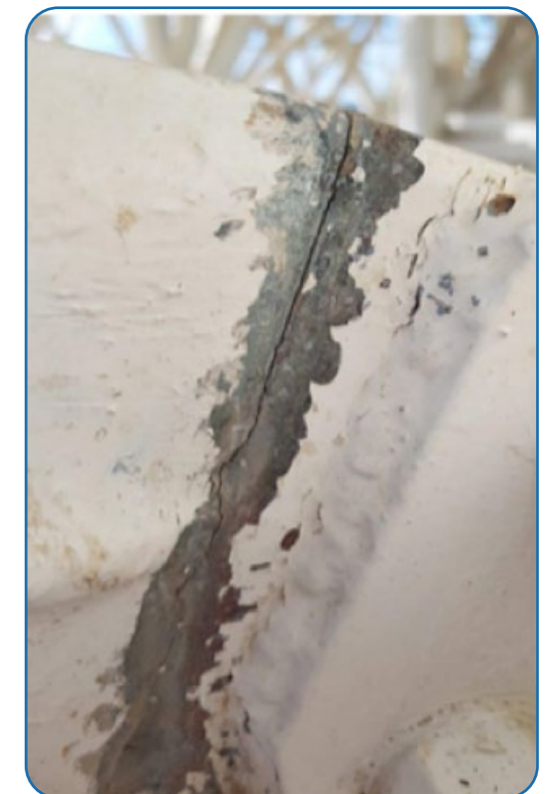
Fig. 1: Crack after the coating removal.
