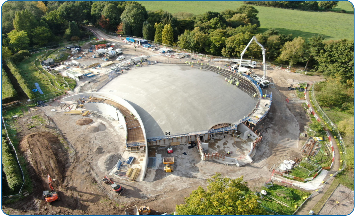
Figure 2. Construction of the Discovery Centre's First Light Pavilion at Jodrell Bank – photo credit Keir Construction
